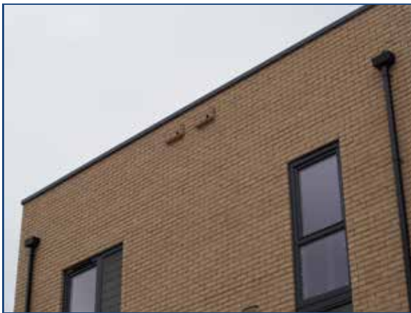
Swift Boxes, Coach House Mews, Bicester (Cherwell Build Project)
